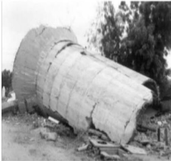
Fig. 3. Collapse of water tank in bhuj
