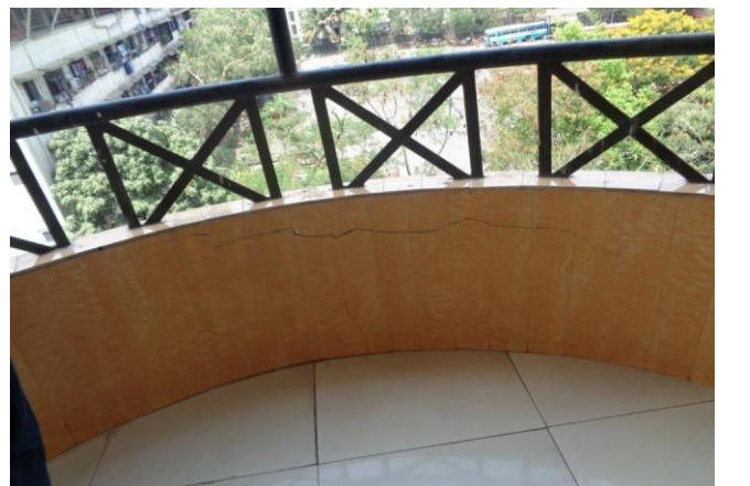
Fig 6: Cracks on balcony Parapet walls.
