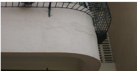
Fig 1: Cracks seen on pardi.
