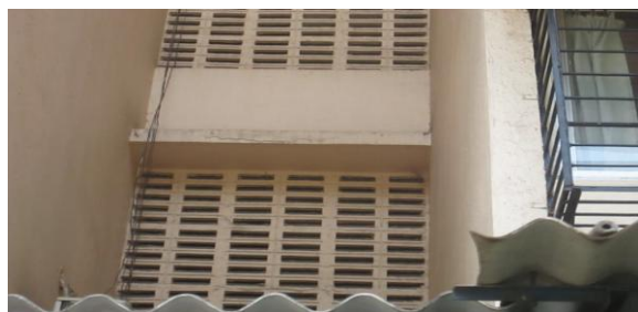
Fig 2: Cracks seen on chajja.
