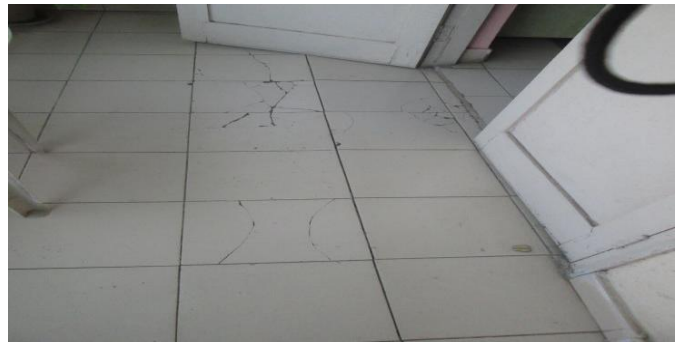
Fig 3: Uplift of tiles due to corrosion
