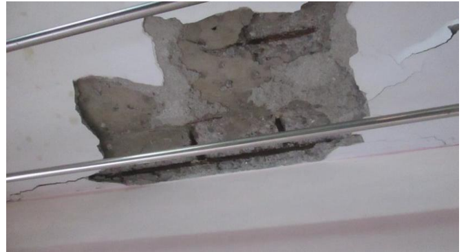
Fig 4: Corrosion seen in slab.
